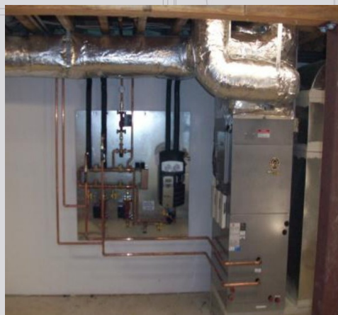
Indoor Fan Coil and Pump station
